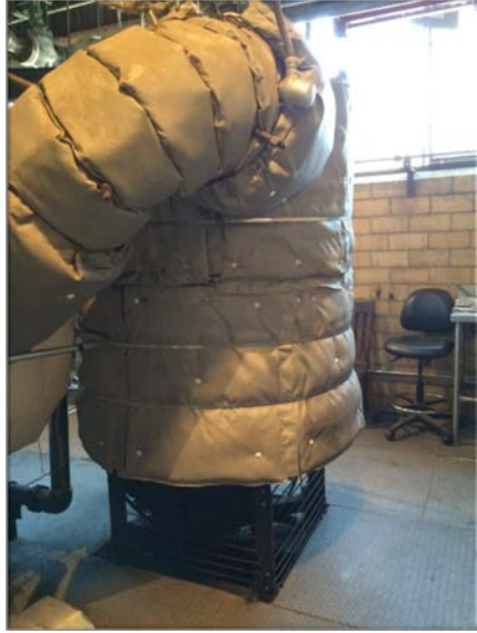
Figure 3.5: Outer view of the gasifier in Oakdale
