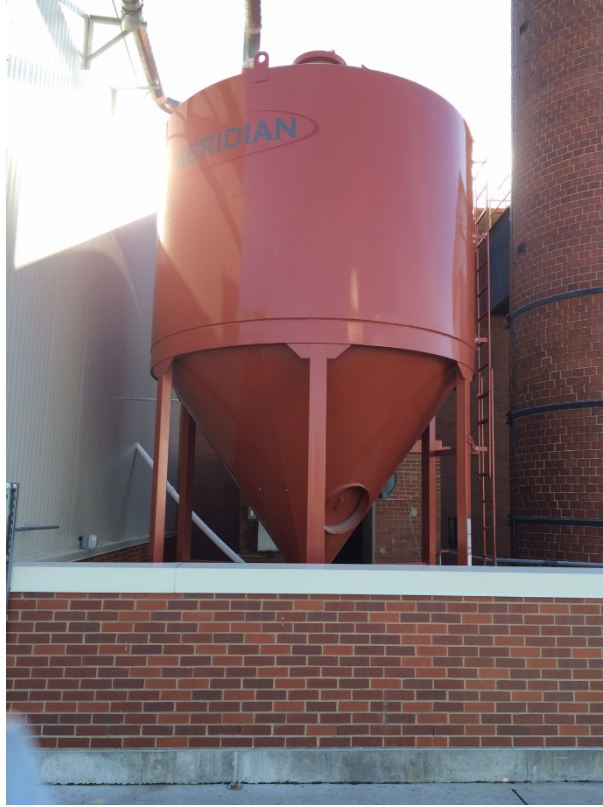
Figure 3.3 Primary Fuel Bin
